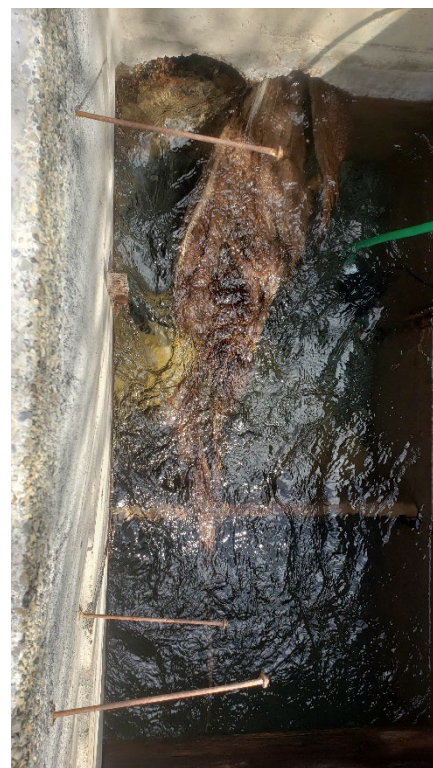
Photo 5-2: Lower Springs Weir Box
