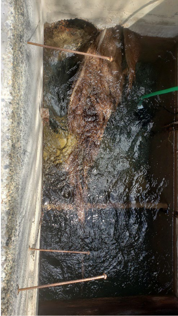
Photo 5-2: Lower Springs Weir Box
